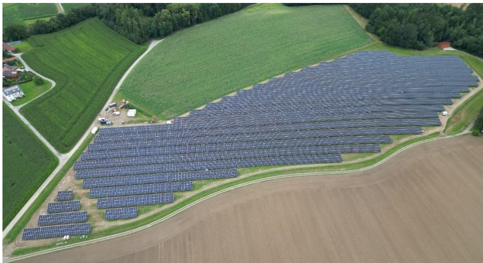
Bürgersolarpark Kraiburg am Inn in Bavaria will commence operations in late 2023. Image: MaxSolar
